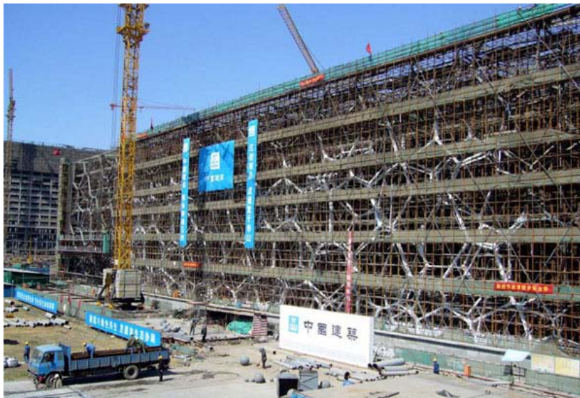
The Water Cube under construction Photo: provided to Sino-US.com by Gilbert Van Kerckhove
