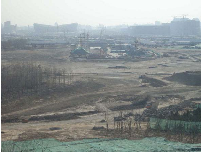
The forest park and lake under construction Photo: provided to Sino-US.com by Gilbert Van Kerckhove
